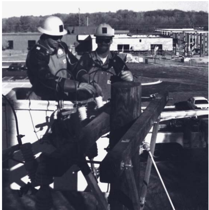
Today's line crews use bucket trucks to work on electric lines, when accessible. Before the 1970's, IPL employees climbed power poles to do the same work.
